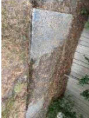
Hazard #46 3117 Bucknell Ct SE bottom of panel is showing, not enough panel to cut
