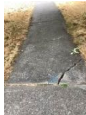
Hazard # 64 Piece is too big to cut, bottom of panel is showing
