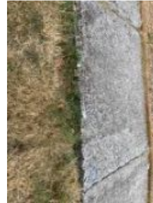
Hazard # 51 3129 Bucknell Ct SE Can see bottom of panel, next to brown fence
